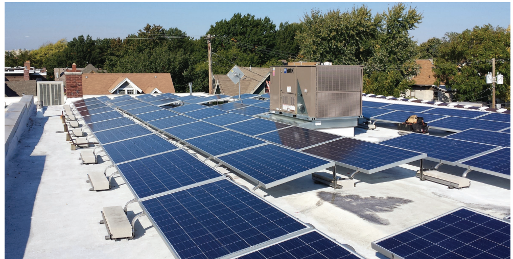
Array of solar electricity generating panels on the rooftop of Arrow's Troost plant.
